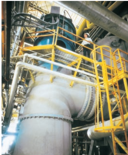
Typical circulating water pump installation
