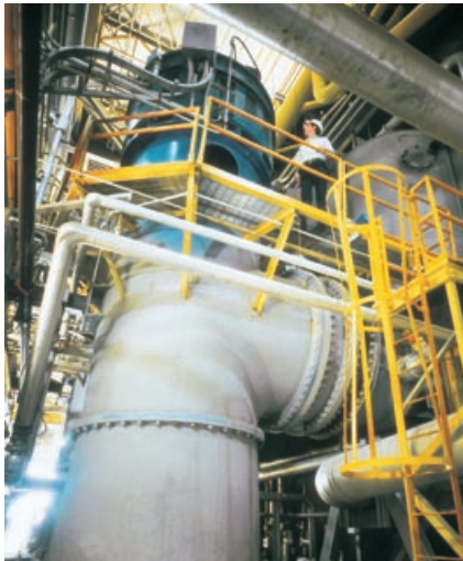
Typical circulating water pump installation
