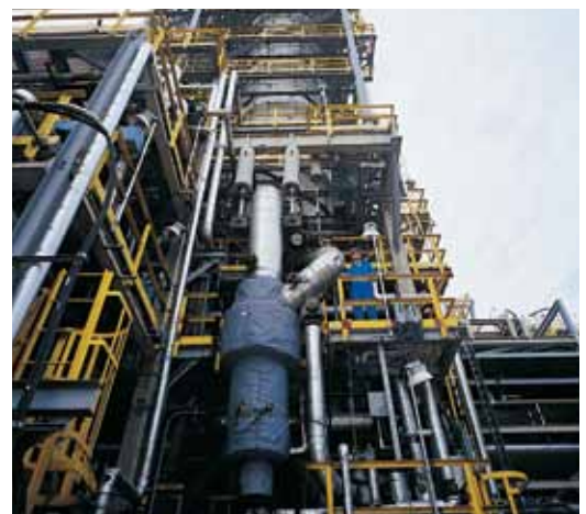
Type PR Reactor Recycle Pump Installation
