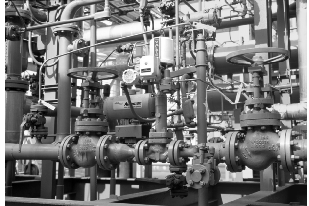
This 2-in Guardian II valve operates in a chemical plant.
