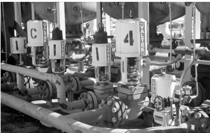
(left) Mark One valves used to operate a PSA skid.
