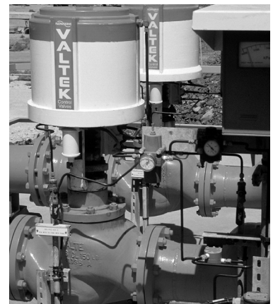
(right) A liquid nitrogen loading facility in Australia uses two Mark One valves for its emergency fire water system.
