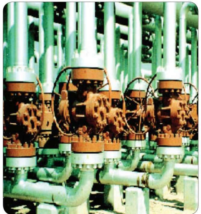
Figure 1b: Onshore manifold with single plug valves
