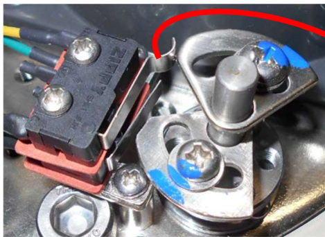
Figure 11: The upper cam is tripping the upper switch.
