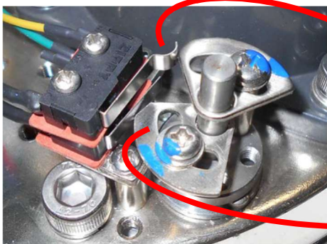
Figure 11: The torque switch cams and switches are shown in the normal operating position.
