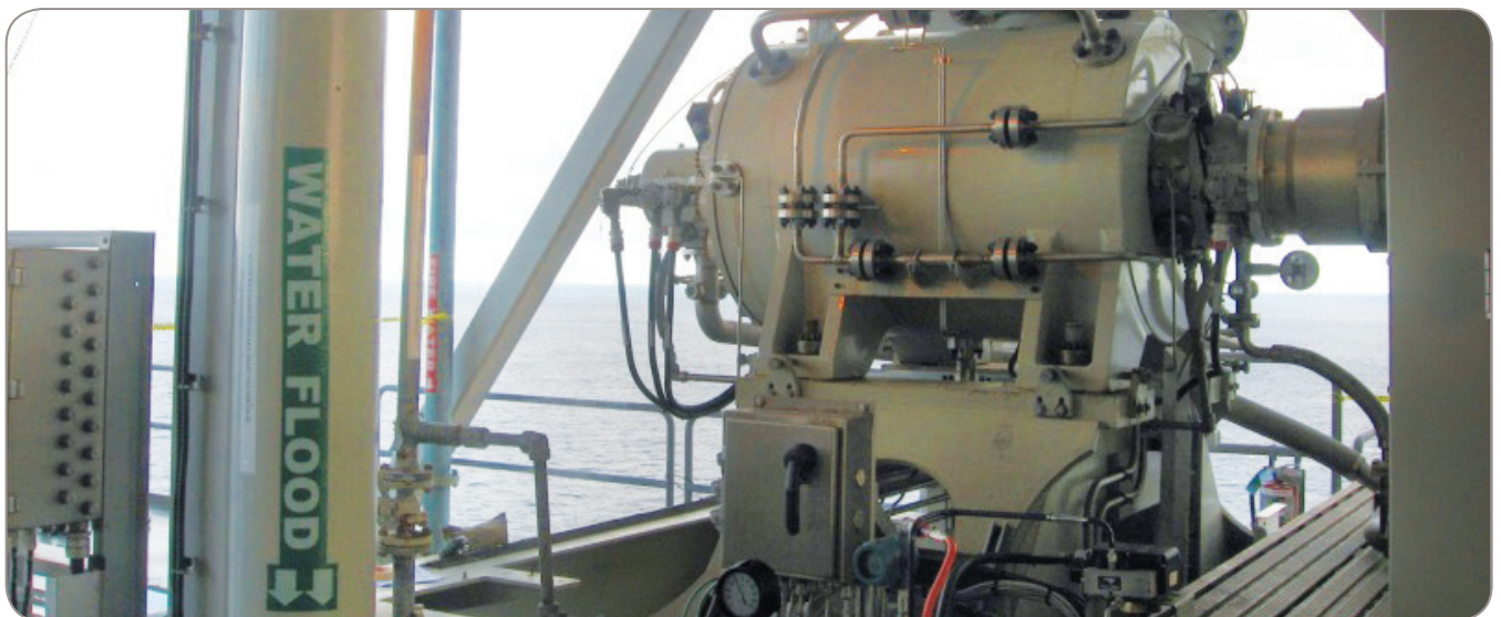
Figure 1: Water injection pump, offshore, CGT drive
