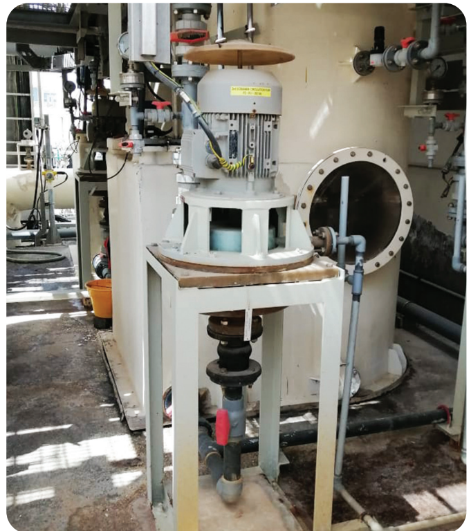
Existing circulation pump installation
