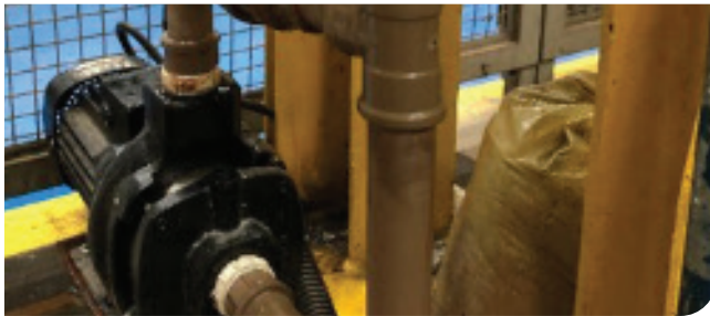
An automated system delivers reclaimed water to the wash cabin.
