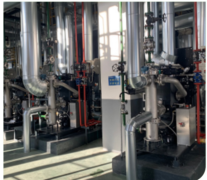
SIHI H1000 Dry vacuum pumps from Flowserve installed in a biodegradable plastics plant in China
