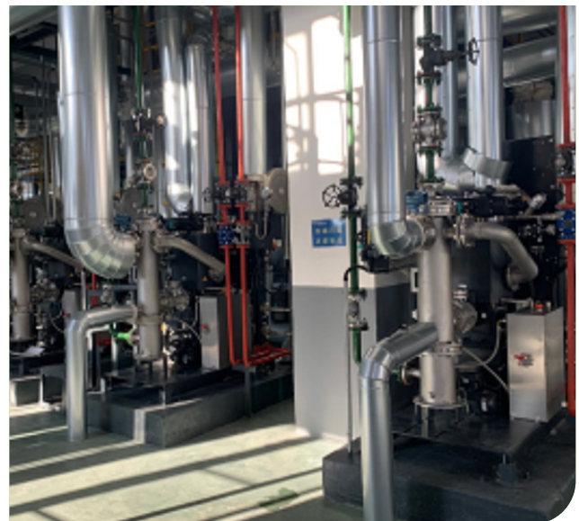
SIHI H1000 Dry vacuum pumps from Flowserve installed in a biodegradable plastics plant in China
